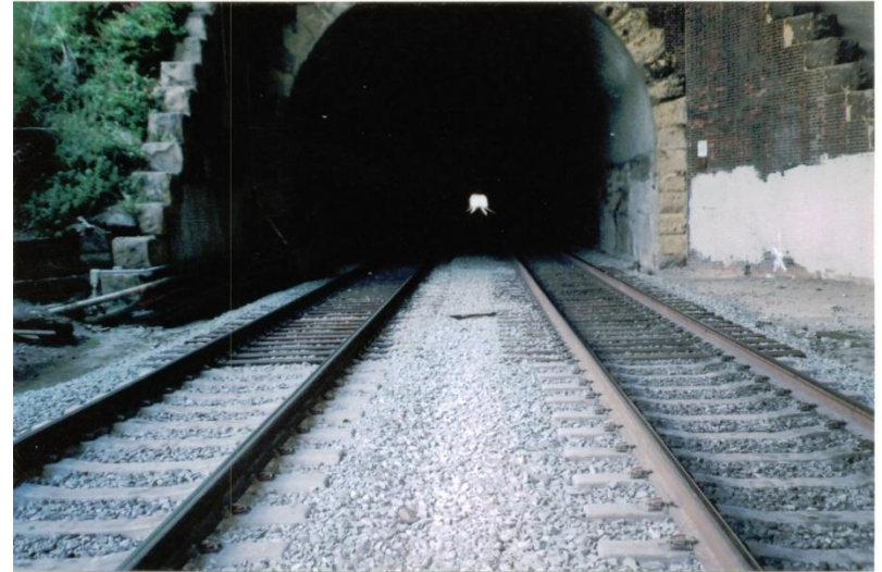
South portal to tunnel #1 from 22 nd Street station, PN 1.9. Asphalt placed in tunnels and approaches during 1999. No surfacing required. Wood ties used in tunnels.
