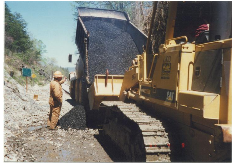
Unloading hot mix asphalt at north end to be distributed by loader
