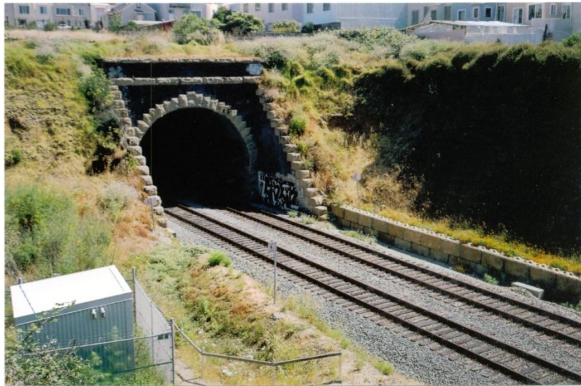
Looking north at south portal to tunnel #3 at PN 2.5. Pumping station at left. All 4 tunnels have sump pump systems. All 4 have asphalt
