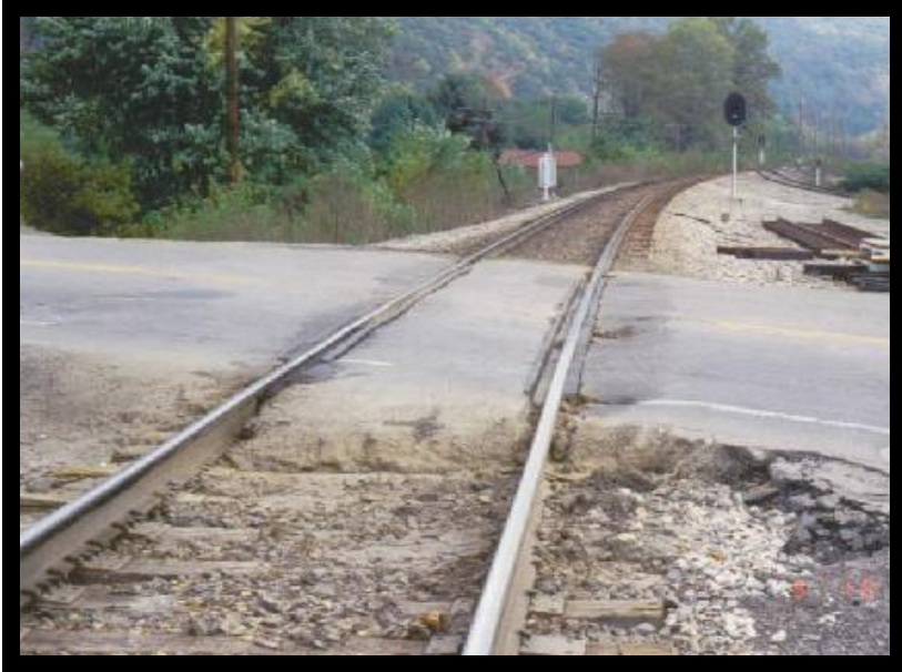
KY 3 Condition prior to rebuild
